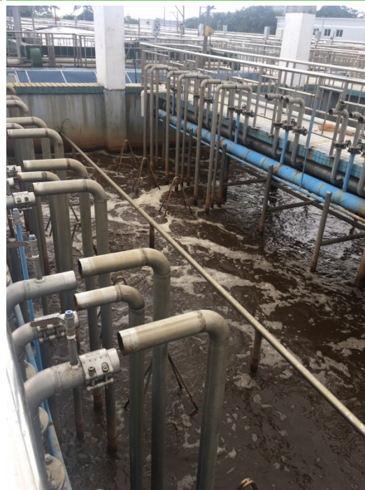
Exhibit 10: Main petrochemical waste water treatment facility
