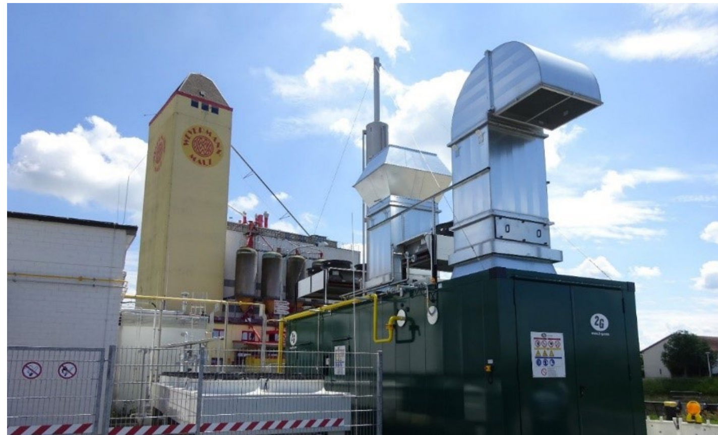
Exhibit 10: 2G Energy installation in Haßfurter Hafen
