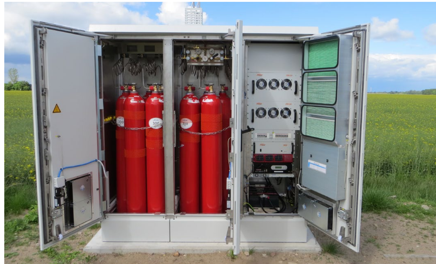
Exhibit 23: Back-up power for BOSNet radio tower sites (hydrogen fuel cell )
